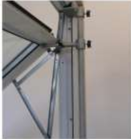
Friction Stay not able to open sufficiently.
